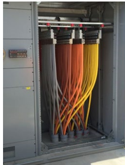
(Color coded 277/480V phasing example with colored secondary conductor installation)
